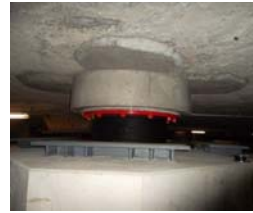
Lead Rubber Bearing with Isolator used
