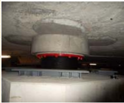
Lead Rubber Bearing with Isolator used
