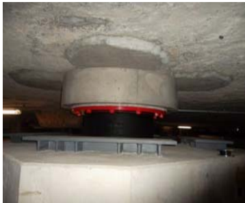
Lead Rubber Bearing with Isolator used
