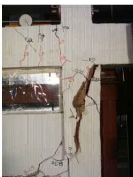
Shear failure of right column
