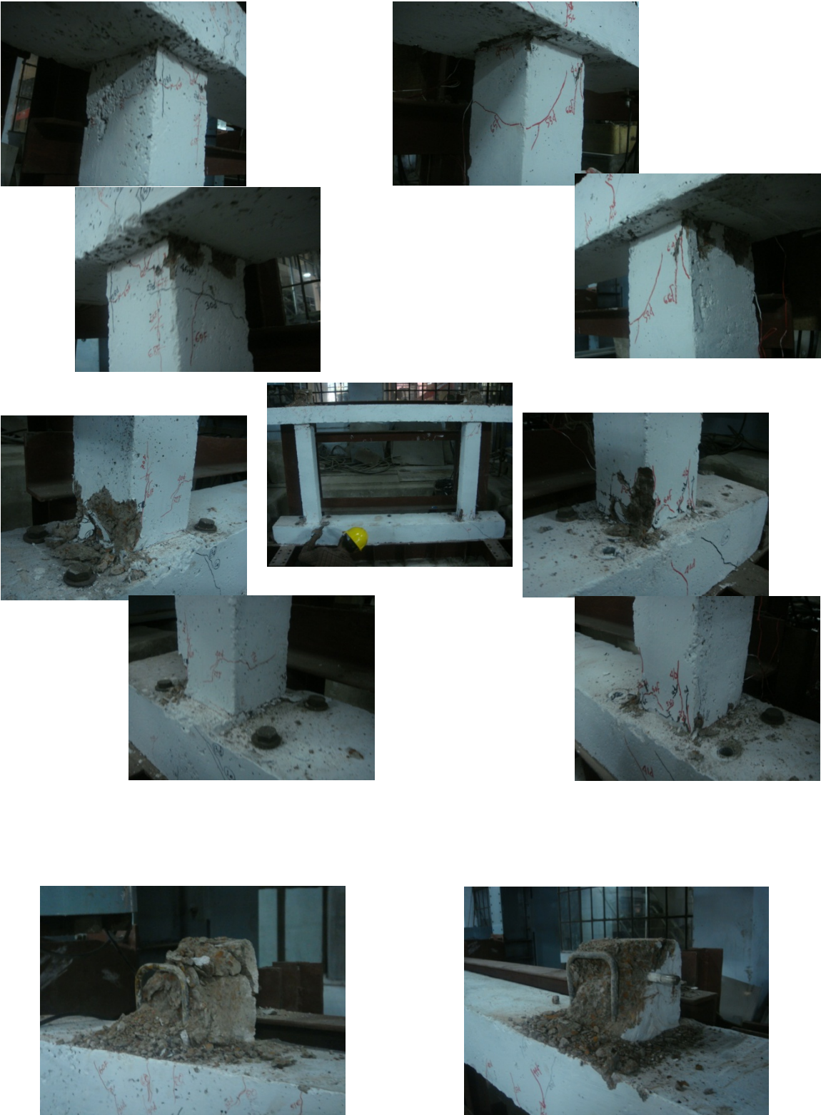
Collapse of column top caused by axial force was observed (after the test). Possible reason is that concrete was weak with honeycomb. This limited the size of vertical loading.
