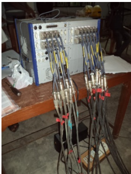
Data logger and connecting cables
