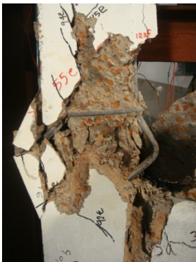
Buckling of main re-bar
