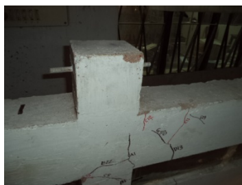
Damage of column top (No.3) was minor after the test.
