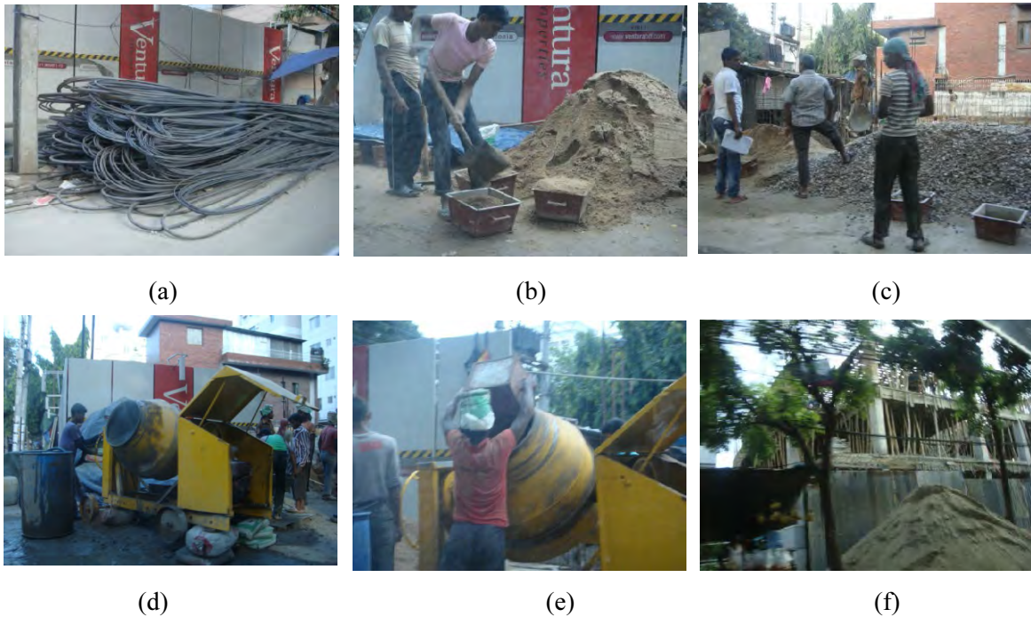
(a), (b), (c) Temporally stocked folded re-bar, aggregate and sand, (d), (e) Mixing by volume, (f) Bamboo support (wearing safety helmets is not common)
