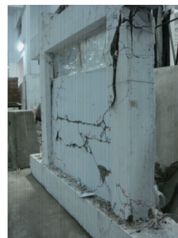
Out of plane movement of brick wall
