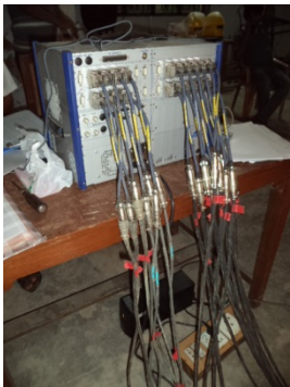
Data logger and connecting cables
