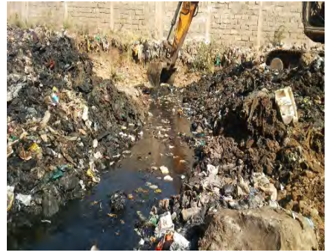
Photo 2-4 Implementation of Drain Installation and Draining off of the Water in the Foundation
