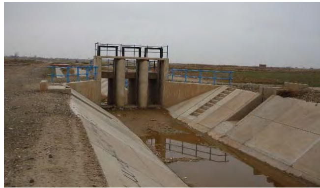
Figure 3.3.1 Irrigation Canal and Diversion Facility of the Under-developed Irrigation System in the Southern Area of Tabriz (in the Aji Chay River Basin)
