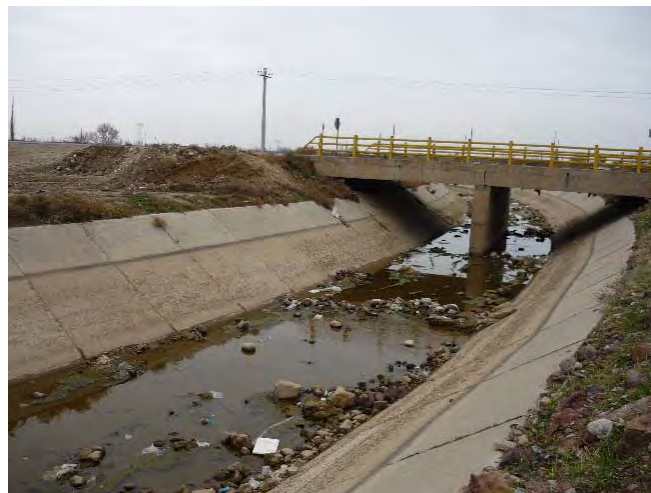
Figure 3.3.2 Irrigation Canal in the Right Bank Area of the Zarinah Rud River, which receives Agricultural Water Supply from Bukan Dam
