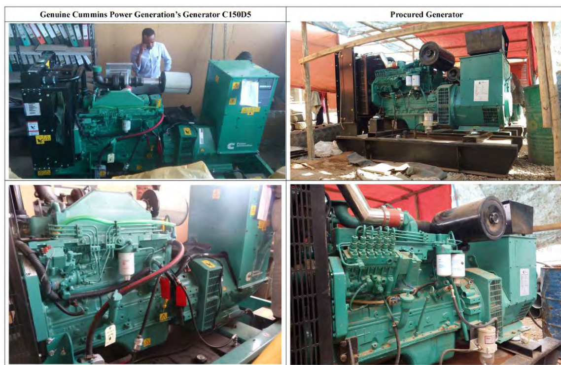
Left photos show the genuine EBG generator while the ones which arrived in Gode shown in right photos show different parts from the original one.
