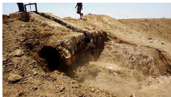
Water leakage from DB No.1 in Ilan; Amount of water leakage increased quickly after starting its leakage, then canal embankment collapsed.
