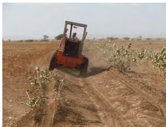
Finally field canal construction started on 14 th February 2014 at the Godiray site with a grader.
