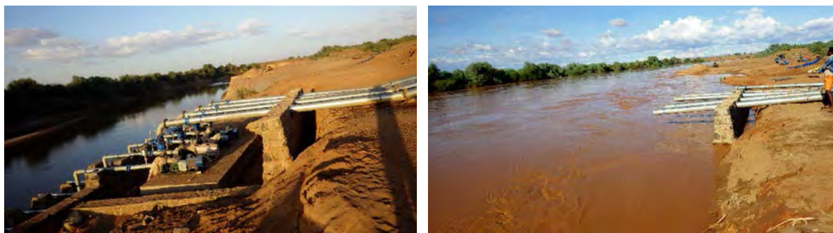
Godiray before and after the flood on March 23, 2015; Water level rose by about 7 m.
