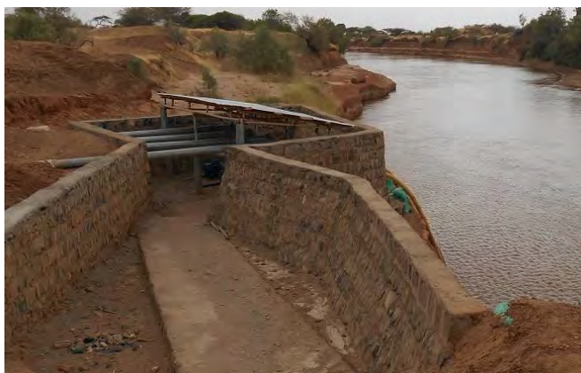
Concrete pavement was constructed for improvement of the access road. In addition, retaining wall was extended and raised for flood protection.
