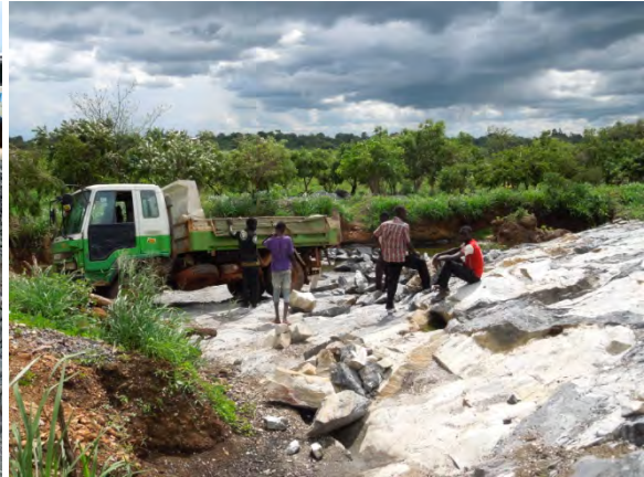
Truck for loading crushed rock
