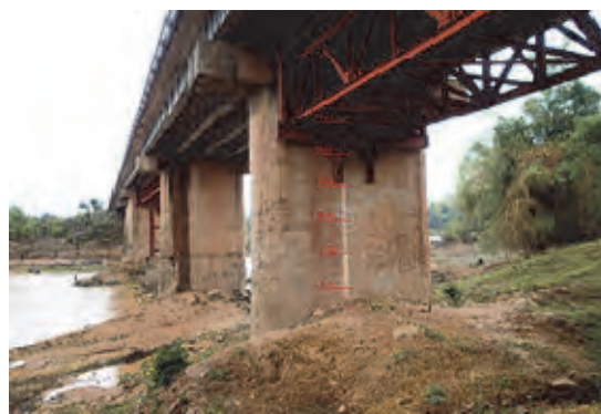
Figure 1.2.35 Trace water level observed in visual inspection
