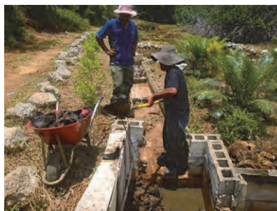
Changing of filtration materials
