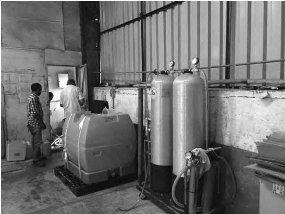
Picture 6.1. Ion-exchange unit for electroplating wastewater treatment installed in Aero Coach
