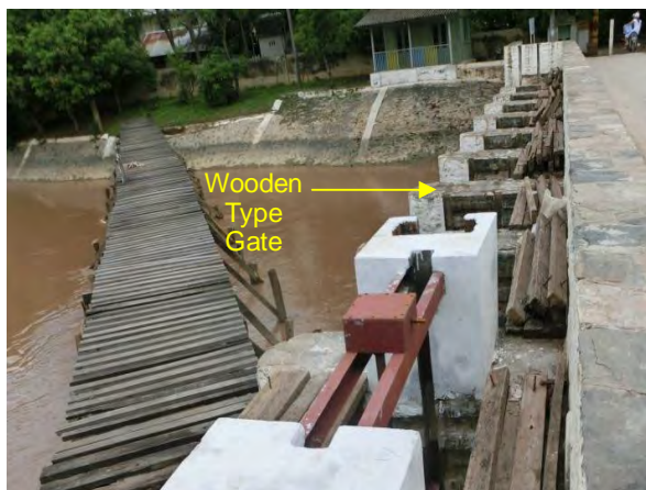
Photo shows the Zeedaw Weir which was constructed in 1890 th . The gate leaf is wooden typed stop log, requiring up-grade to steel leaf.
