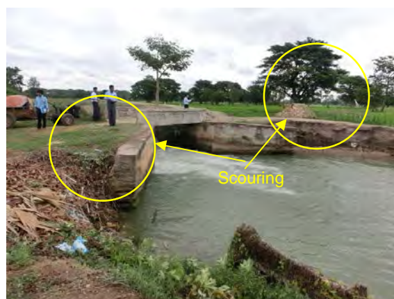
At the downstream of a hydraulic structure in a DY canal in SMC, it is found that both sides of the embankment have been scoured by water flow. Protection for embankment is needed.
