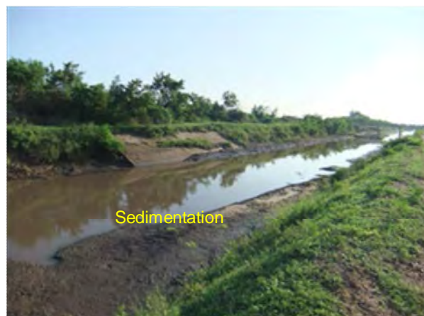
At the Kinda Left Main Canal, the sedimentation reduces the capacity of canal and causes the water shortage in the downstream command areas.
