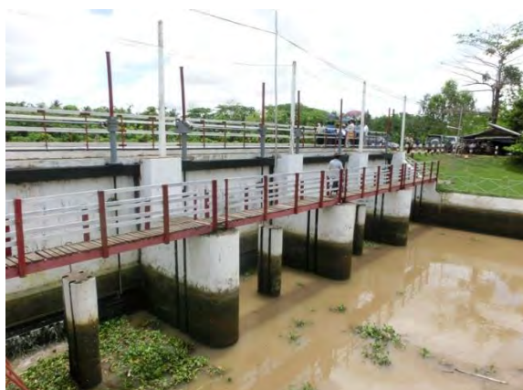
Photo shows the sluice gate for preventing the saline infiltration through drainage canal. Some parts of gate are deteriorated and there is leakage through the gate.
