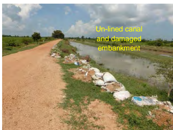
Photo shows the un-lined canal which is located along OMC. The un-lined canal damages the inspection road and weakens the canal embankment.
