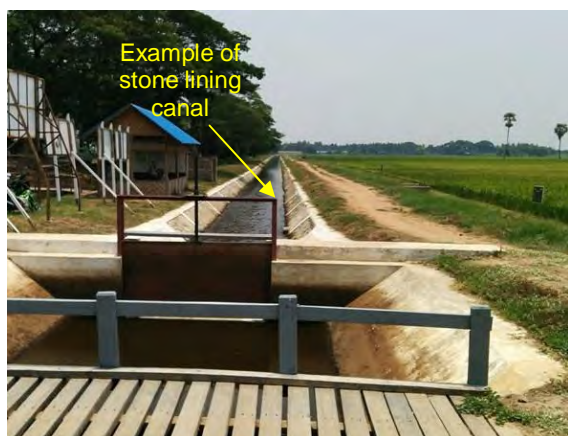
Photo shows the example of upgraded canal by stone lining along a secondary canal of Yezin Irrigation System. The upgraded canal contributes to the reduction of water loss from the canal bank and bed.
