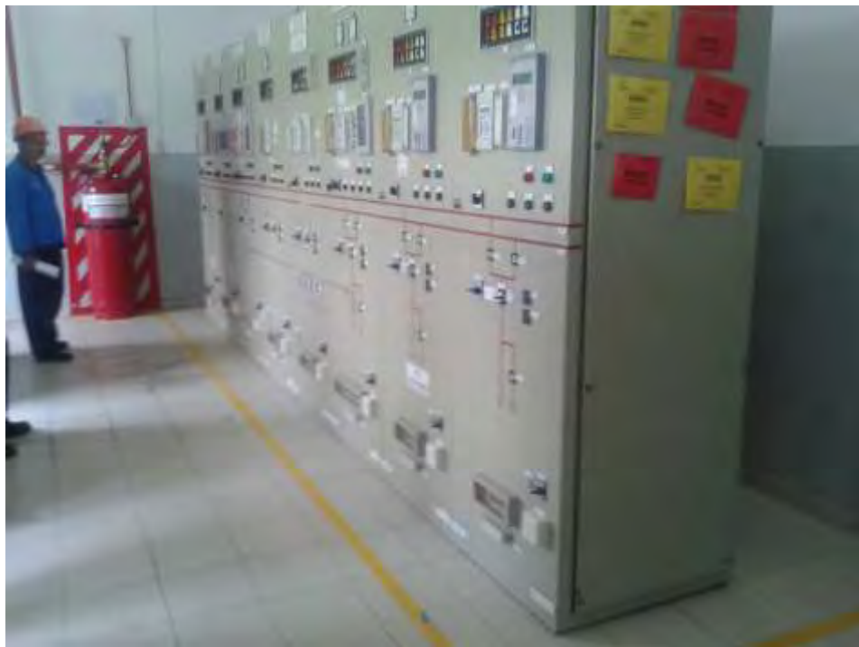
Figure 4: 33kV Control Panel in PMU Kangar
