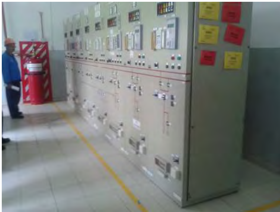
Figure 4: 33kV Control Panel in PMU Kangar
