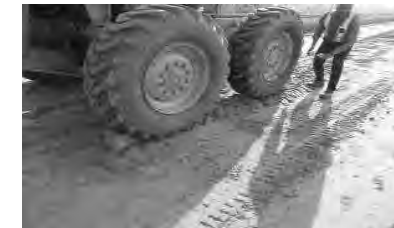
Chocks available for grader. This are not being placed in consistent locations under wheels This should be standardized across the project
