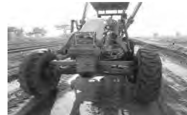
The grader operator was working without clear demarcation of the work boundaries. Safety Cones and florescent tape should be used to clearly mark the safe working area
