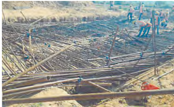
Figure 4.3.6 Vertical Steel for Side Wall of Box Culvert Collapsed by Strong Wind
