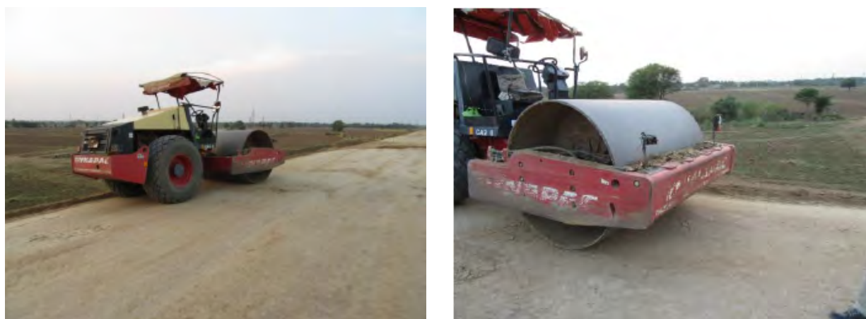
Figure 4.3.20 Accident Site and the Compaction Roller
