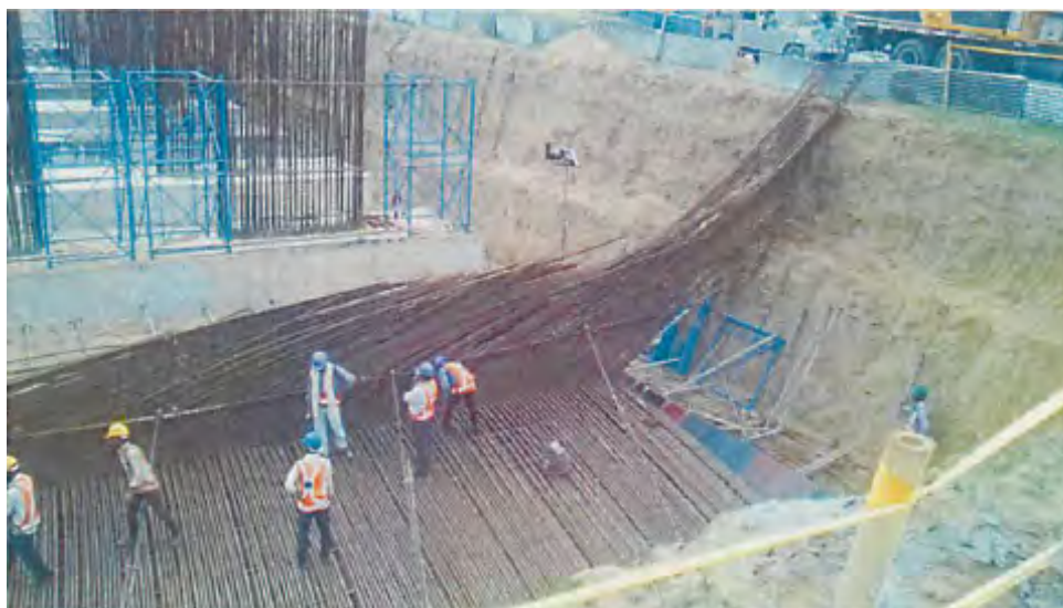
Figure 4.3.1 Vertical Steel for Abutment Wall Collapsed by Strong Wind
