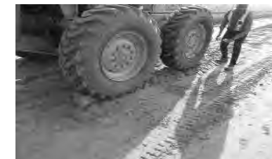
Chocks available for grader. This are not being placed in consistent locations under wheels This should be standardized across the project
