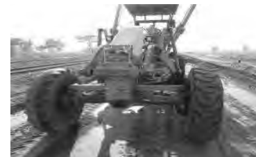
The grader operator was working without clear demarcation of the work boundaries. Safety Cones and florescent tape should be used to clearly mark the safe working area
