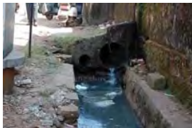
Existing condition of Drains
