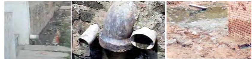
Figure 21: Discharge of Grey Water in Drains
