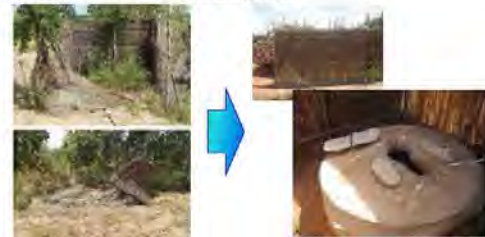
The existing latrine consisted solely of a structural frame, which was made of mud bricks.
