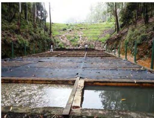
Leachate treatment facility
