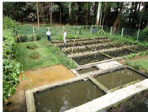
Toilet waste treatment facility
