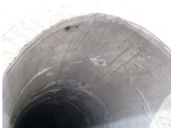
Tunnel No.3 (lighting) (2014.6)
