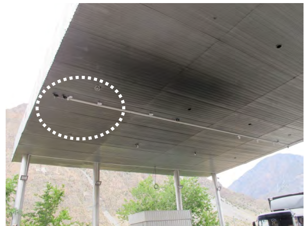
Kara-Kyol toll gate (Camera type)
