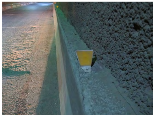
Delineators (experimentally installed)
