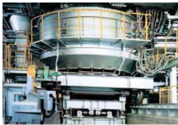
Ash melting facility
