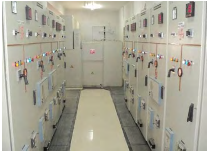
Appendix 16: Use of IT in Substation: Torrent Power (Agra)
