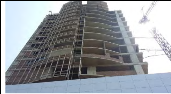
9: High rise building in Lahore Reinforced Concrete structure with curtain wall facade are under construction.
