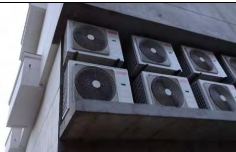
16: AC condenser at retail buildings Majority of AC system is split system that installed by tenant owner.
