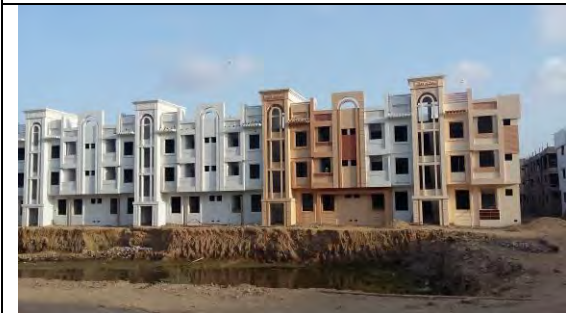
11:3 storey apartment in Karachi Windows will be installed after completion of wall plaster and finish. Air-tightness is an issue.
