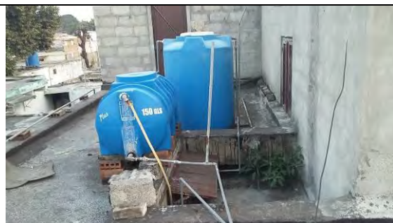
14: Water Tank on top of roof Pumped up from public supply water pipe by each house owners.
