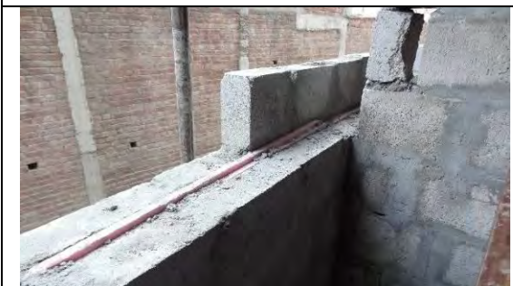
13: Heat insulation on wall 2 inch insulation (XPS) sandwiched with 4 inch double concrete block wall.
