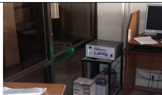
24: Office with UPS
