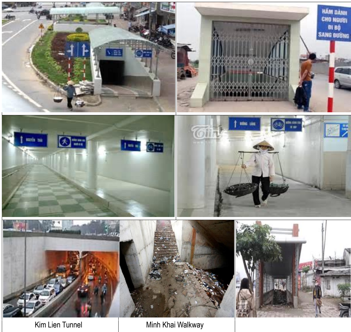
Figure 2.2.4 Condition of Pedestrian and Vehicle Tunnels
