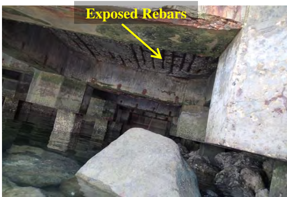
Figure No.4 Under deck slab and beam of the old RC Pier.
