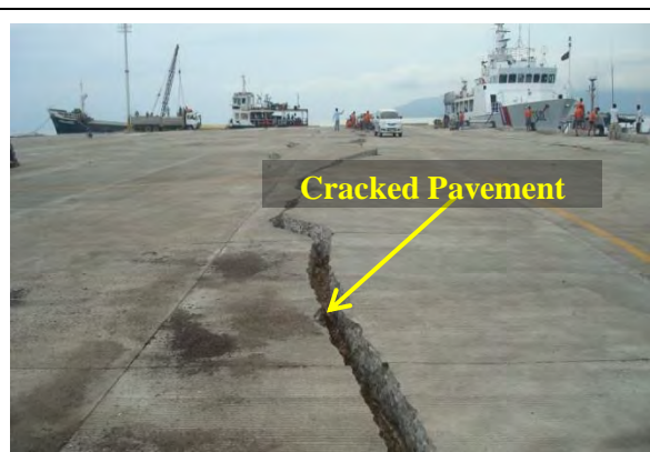
Figure No.3 Damaged after OCT 2013, 7.2 magnitude EQ.
