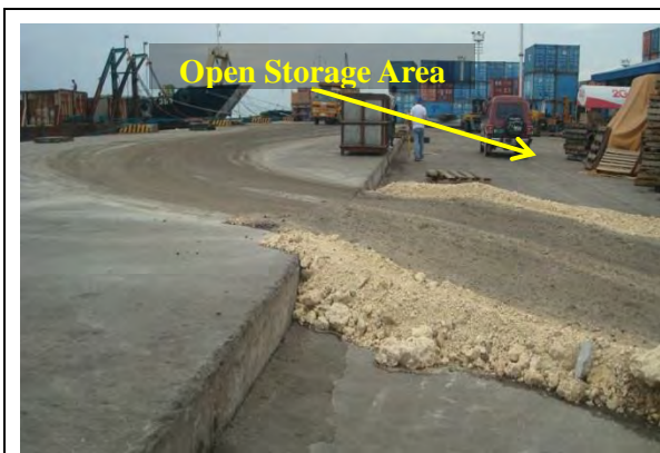
Figure No.2 Concrete Pavement at Open storage area settled after the OCT 2013, 7.2 magnitude EQ.
