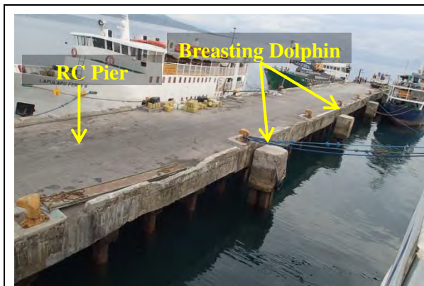
Figure No.2 The figure shows the Northwest (NW)/ right side of RC Pier
