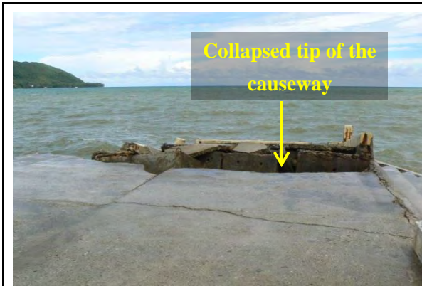
Figure No.4 Collapsed portion of the Causeway due wave action.
