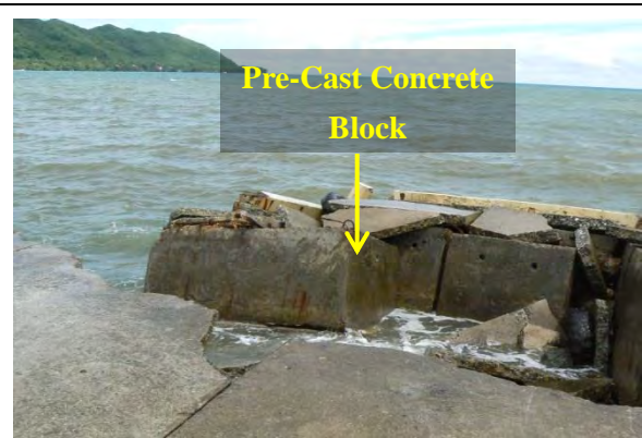
Figure No. 5 Exposed Pre-Cast Concrete block of the collapsed causeway.
