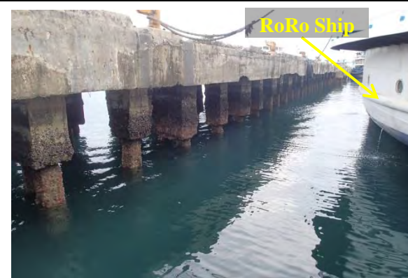
Figure No.5 The concrete pile of RC pier near the RoRo ramp.
