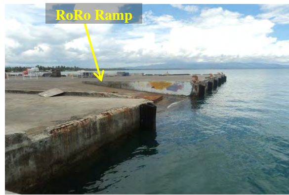
Figure No.5 The RoRo ramp at the east side of the port during high tide.
