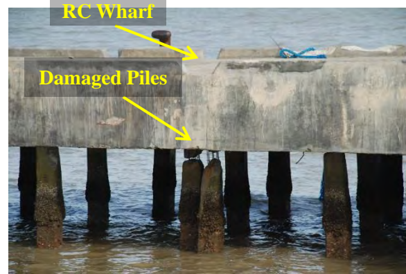
Figure No.3 Damaged RC Piles under RC Wharf.
