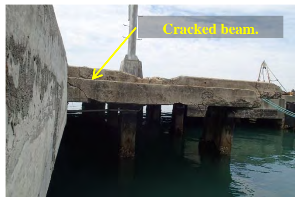
Figure No.7 Portion of the old RC Pier with structural damages visible.
