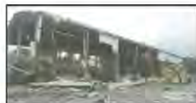
Damaged transit shed by storm surge
