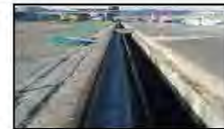
Damaged precast slab by Tsunami in Japan
