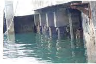
Part of conc. decks and pile caps were damaged by Typhoon and repaired in 2014
