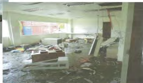
Admin. Office after the typhoon.
