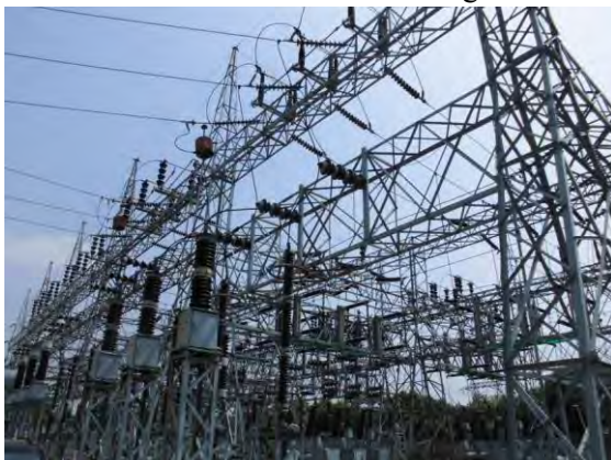
(a) Existing 132 kV Air insulated switchgear
