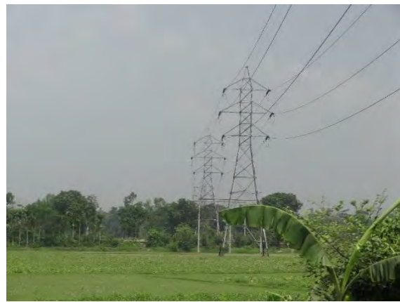
Existing 132 kV Transmission Line
