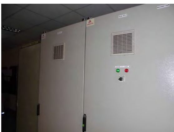
(c) Existing Remote Terminal Unit (RTU) Panel
