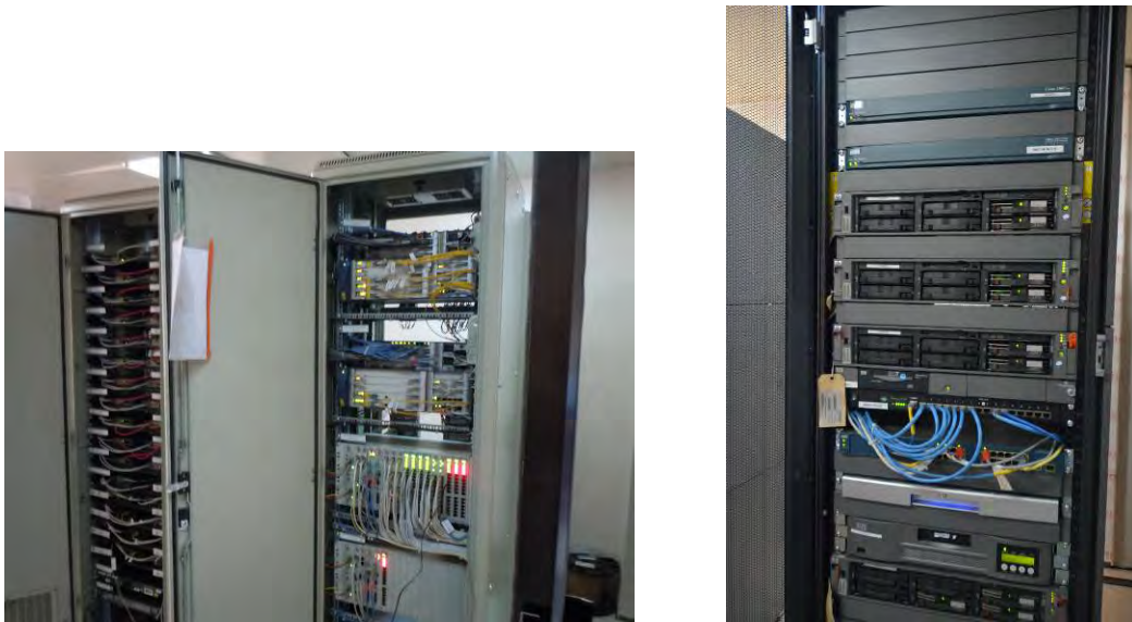
Server and storage
