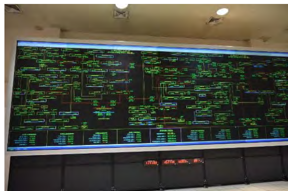
System Monitoring Panel
