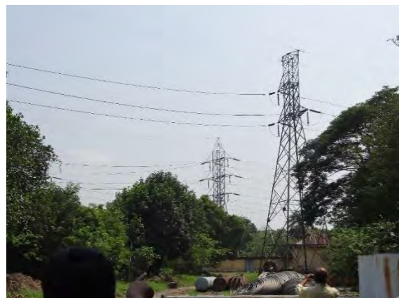
Existing 132 kV Madunaghat SS
