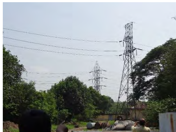
Existing 132 kV Madunaghat SS
