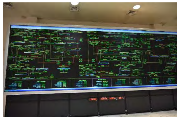
System Monitoring Panel
