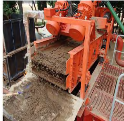
Soil Separating Plant
