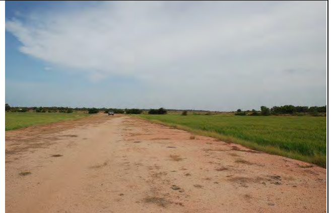
Plate 90. The end of the ring road after the damaged bridge at Mullipotana- Soorangal road
