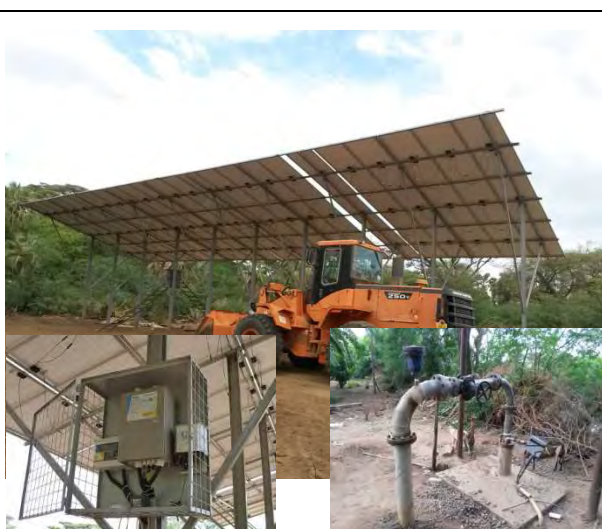
Solar Power Pump System – LOWASCO (Turkana)
