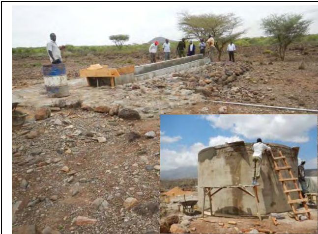
Pipeline System – Arapal (Marsabit)
