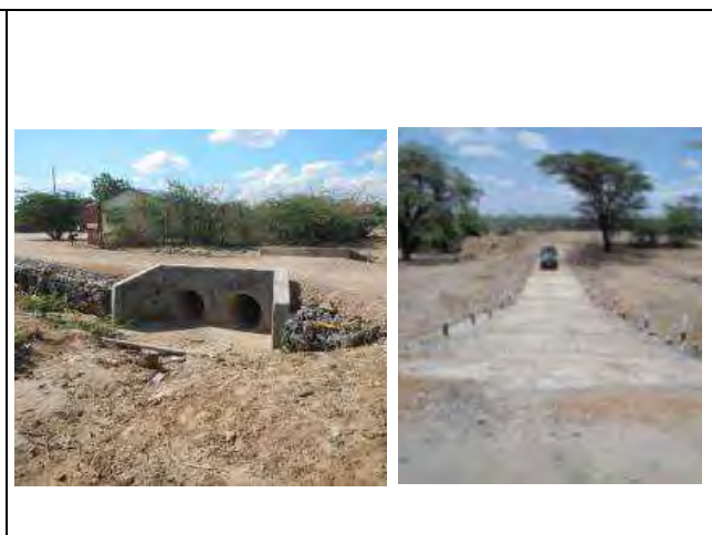
Rural Road Improvement - left: Kakopito drift, right: Lodwar livestock market culvert (Turkana)
