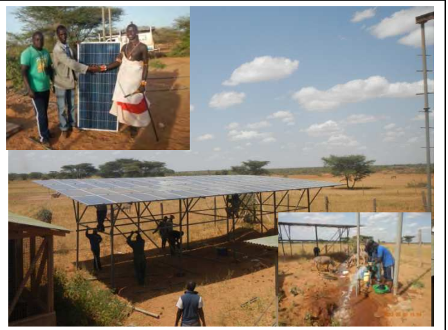
Solar Power Pump System (Marsabit)
