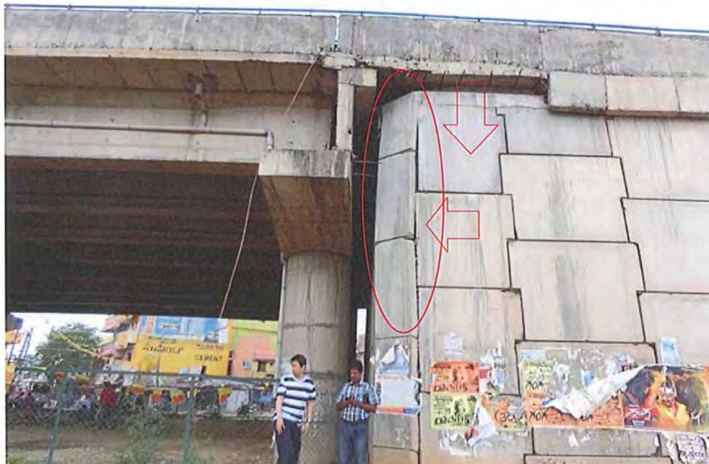
(Deformation at MSE Wall of NH-7 in Bangalore)
