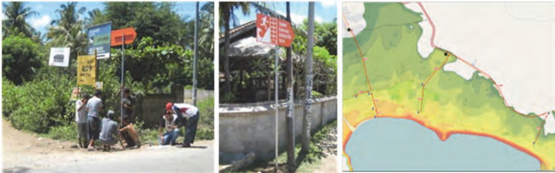
Picture 2.6.15 Installation of Tsunami Evacuation Signboard (Left and Center)/Locations of the Sign Boards (Right)
