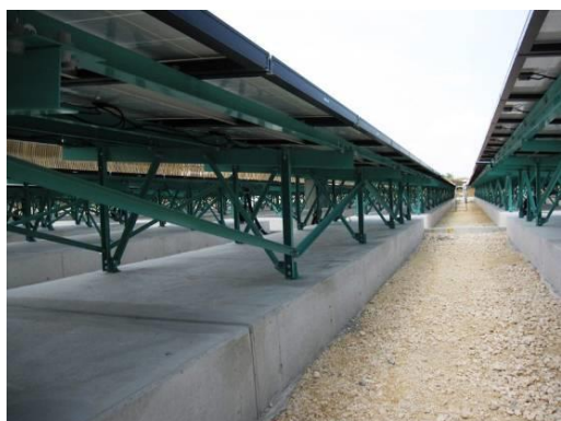
Figure 3-10 Concrete slab foundation (Miyako Island Mega Solar Experimental Study Facility PV foundation)
