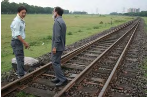
Four (4) rail configuration track is on the bridge.
