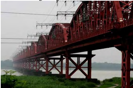
Completed in 1915. One span is about 110m. Well-maintained and last painted in 2012. About 280m downstream, there is the Lalon Shah Bridge which has almost identical span lengths as the Harding Bridge.
