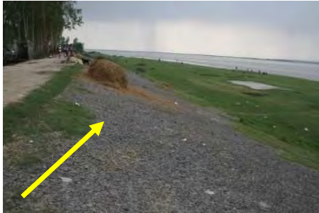
Revetment is here. Sand deposits in front began to be eroded.
