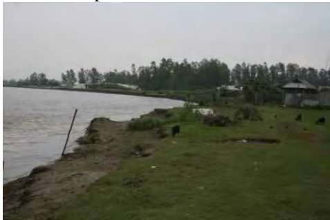
43. Erosion upstream of East hard point and houses on sand deposit
