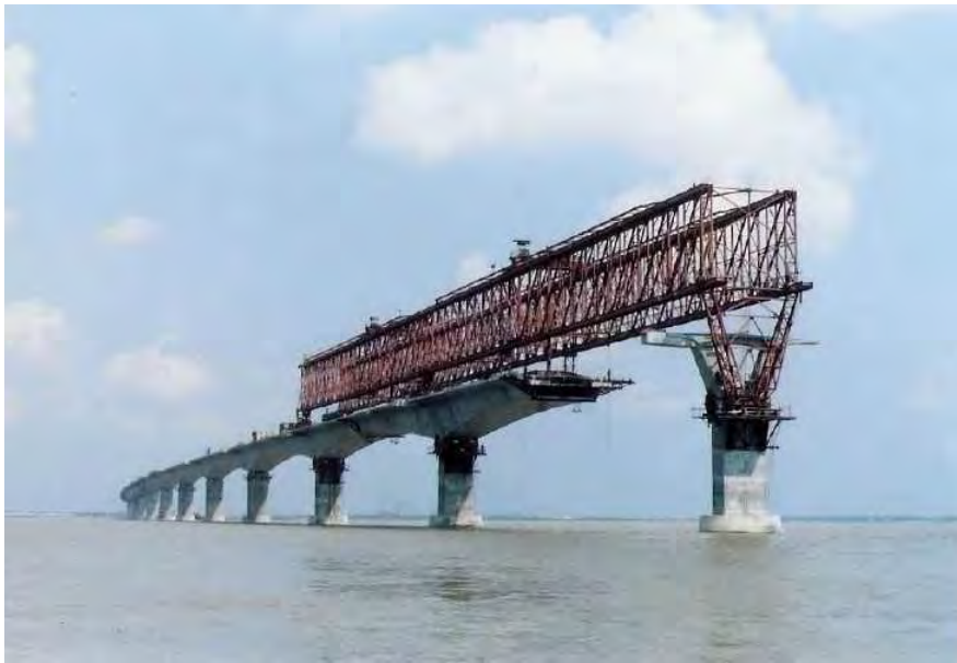
Source : http://www.panoramio.com/user/703267?comment_page=1&photo_page=3&show=best [Fig. 4.1.3] Construction of the Bangabandhu Bridge by the P&Z method
