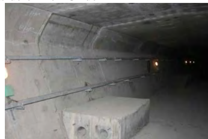
White lines on haunch indicate cracks.
