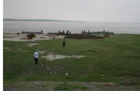
Due to river width reduction at the Bangabandhu Bridge site, some places upstream are attacked by river flow harder. BBA protects such places by sinking sandbags.
