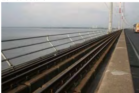
On approach sections three (3) rail track is placed. Only on the bridge section, four (4) rail track is placed. About 300m gap between outer rail and inner rail, which is too large to prevent derailment.
