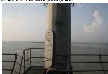
No.26 power line pole is placed exactly above No.26 pier. Poles are also spaced 100m interval.
