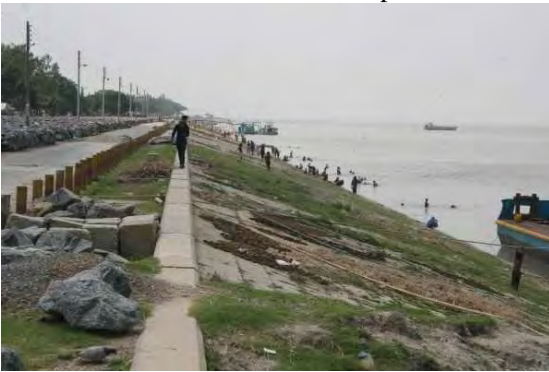
This year no damages on revetment. Last year there were small damages and they were repaired.
