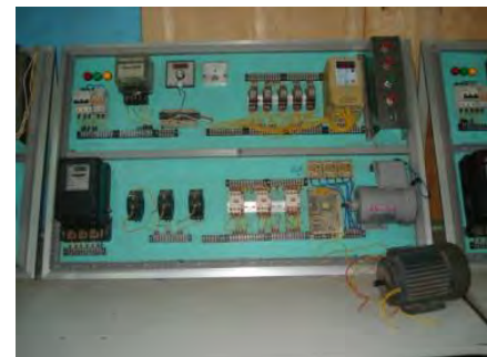
Photo 9-4: Power distribution/panel board devices
