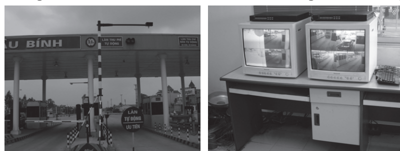
Figure 5.37 Tollgate Lanes and Monitor Screen at Binh Bridge in Hai Phong Province
