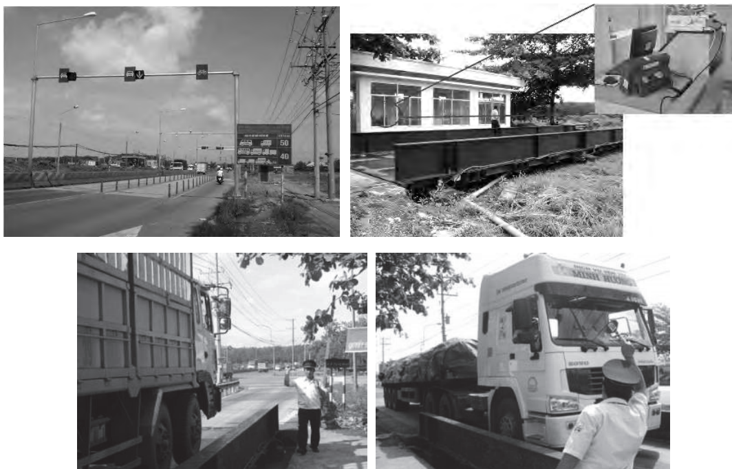
Figure 5.62 WIM System (Left) /Static Weigh System (Right) /Static Weighbridge (Below)
