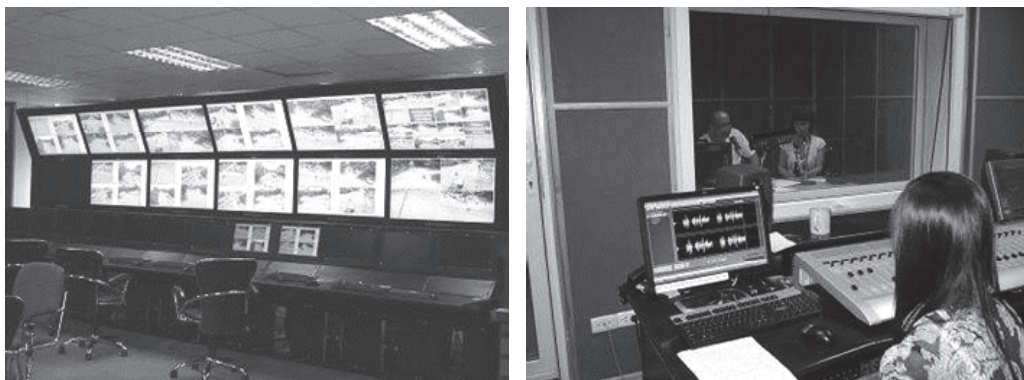
Figure 5.32 Traffic Monitoring Center and Sound Recording Room
