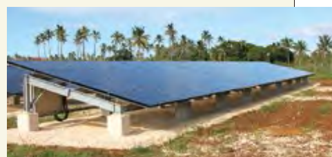
A solar power generation facility in Tonga
