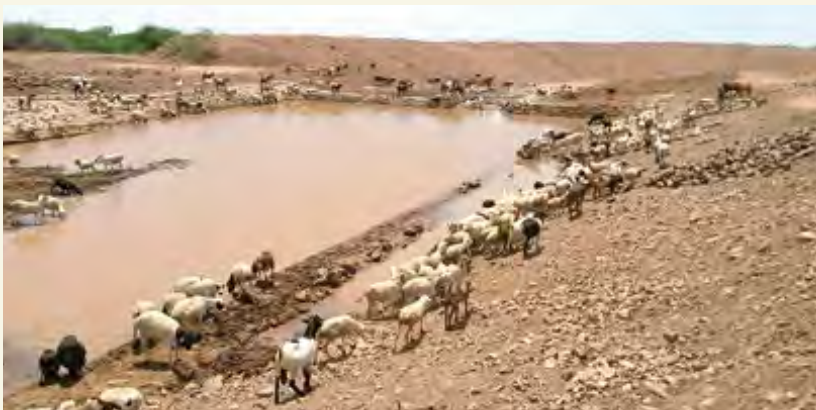
A total of 11 livestock water points have been constructed or improved. These JICA-made “oases” can supply water to many head of livestock even during the dry season or drought.
