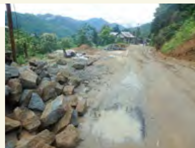
National highway in a northeastern state damaged by severe rain
