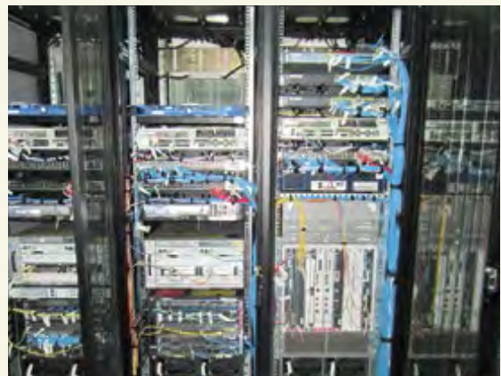
Communication equipment deployed in this project contributed to improving the communication environment in Myanmar.
