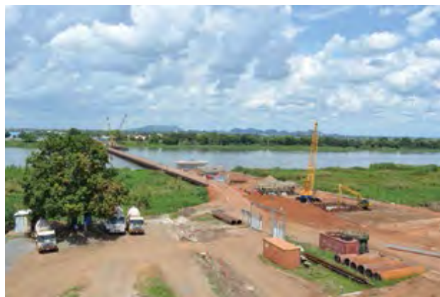
A new bridge over the Nile River under construction. Cooperation resumed on a full scale in South Sudan and the construction of the Nile River Bridge (Freedom Bridge), the symbol of peacebuilding, was also resumed in March 2015. (Photo credit: Dai Nippon Construction)
