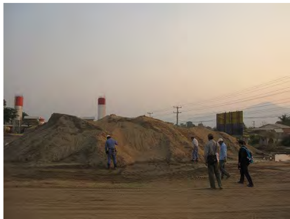
Concrete Mixing Factory at Pakse
