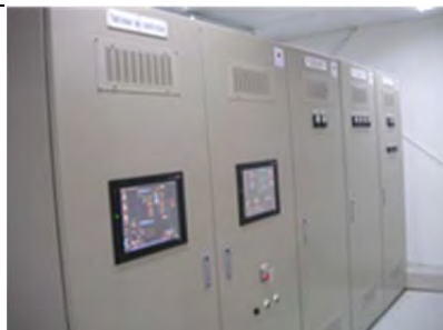
Photo 40 Power control panel
