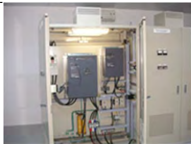
Photo 39 Power control panel
