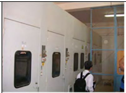
Photo 8 Control panels in the power receiving room
