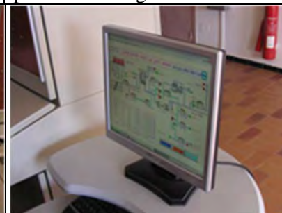
Photo 11 Monitoring display system
