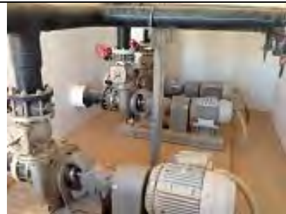
Photo 35 Filter pump, backwash pump
