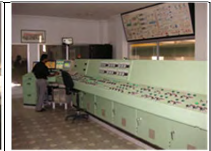
Photo 19 Monitoring operation panel
