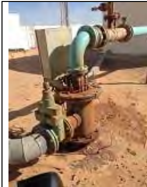
Photo 34 Intake deep well
