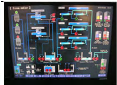
Photo 41 Monitoring display system
