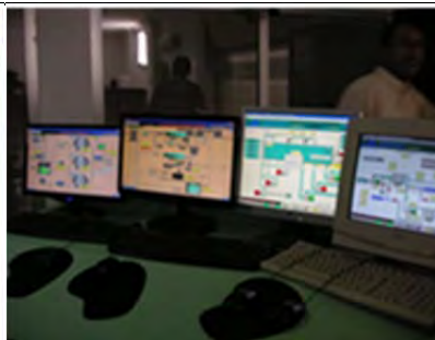
Photo 21 Monitoring display system
