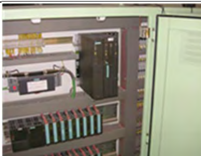
Photo 20 Monitoring operation panel
