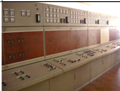
Photo 9 Monitoring operation panel
