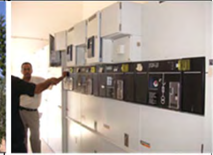
Photo 16 Control panels in the power receiving room
