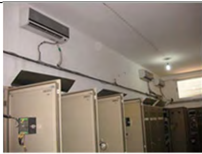
Photo 18 Low-voltage electrical room
