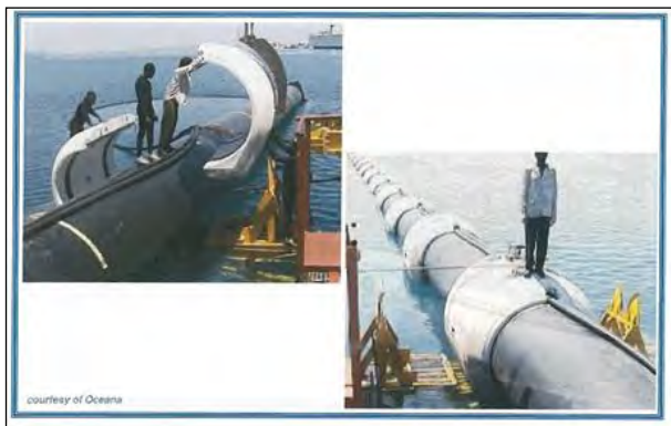
Source: GWI Figure 5.5-3 HDPE Pipe with Ballast Weight
