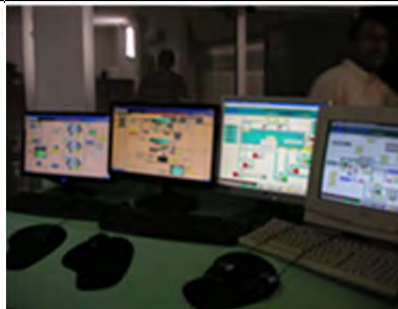
Photo 21 Monitoring display system
