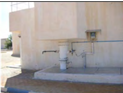
Photo 17 Intake flow meter
