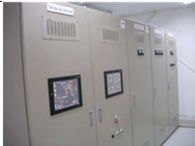
Photo 40 Power control panel
