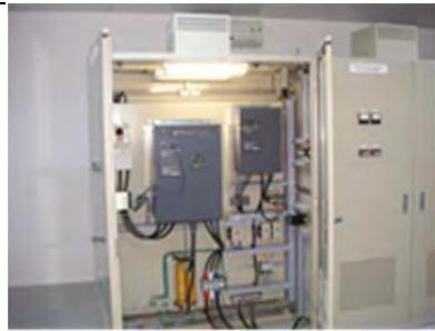
Photo 39 Power control panel
