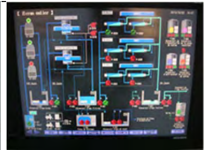
Photo 41 Monitoring display system
