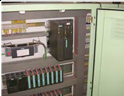
Photo 20 Monitoring operation panel
