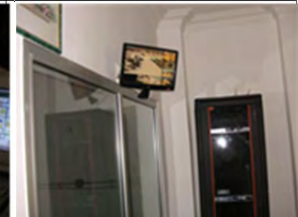
Photo 22 Security camera monitor
