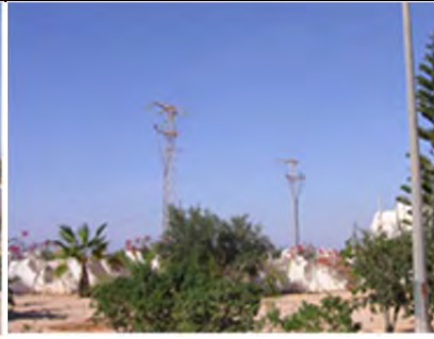
Photo 15 STEG transmission tower
