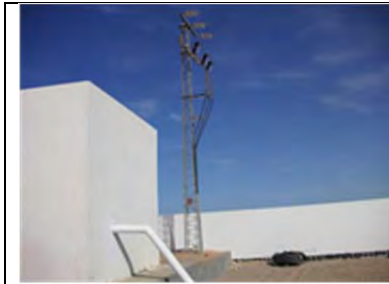
Photo 36 STEG transmission tower
