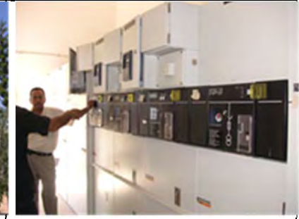
Photo 16 Control panels in the power receiving room
