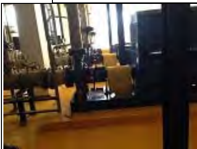
Photo 3 High pressure pumps for RO
