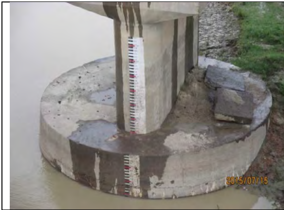
Staff Gauge at Banibad Water Level Station (Bagmati River)
