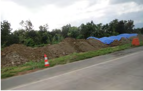
Photo 2.2-2: Excavation site along the STAR Tollway, located on the pyroclastic flow plateau, where partially-consolidated tuff or volcanic ashes are distributed. The excavation site is under the “dry” environment with the groundwater level low.
