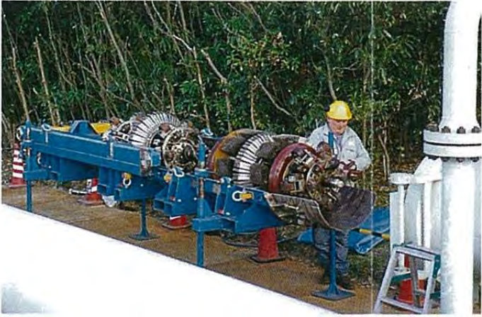
Figure 2.4-24 Inspection of pipeline integrity by Intelligent Pig (Example )
