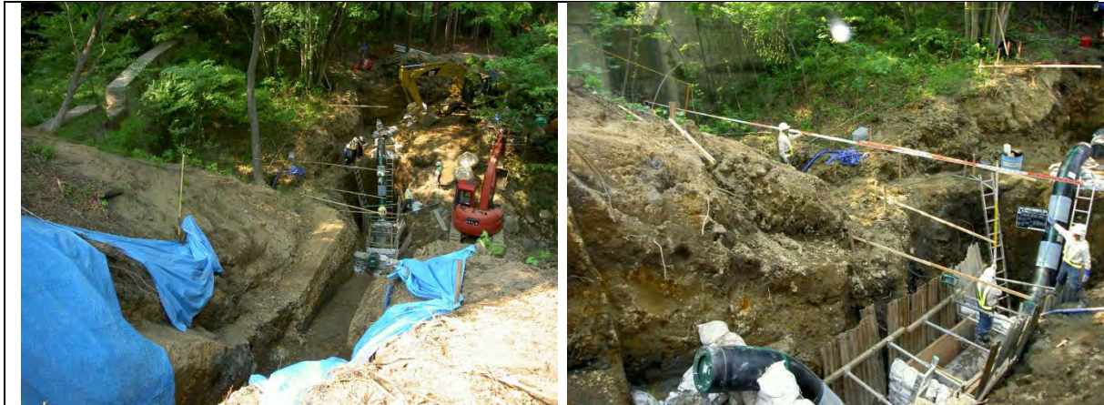
An example of construction work for pipeline installation at a river crossing (a case in Japan)
