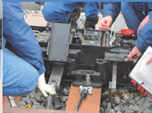
Replace training of electric point machine at the signaling maintenance depot
