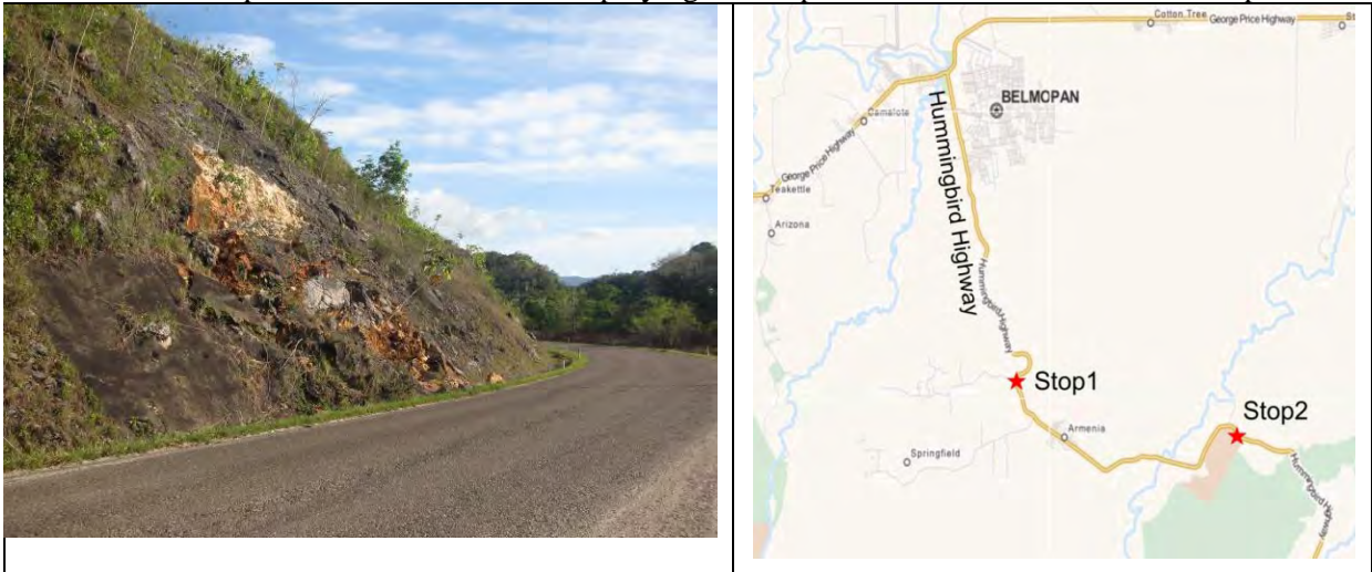
Date: April 6, 2015 Location: Stop 1 – Slope Failure Site Description: Small slope failure site on Hummingbird Highway. Source : JICA Study Team
