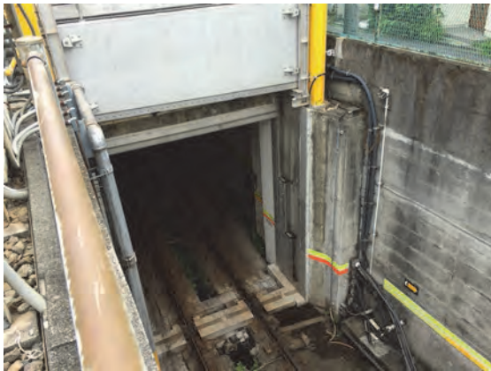
Flood Protection Gate
