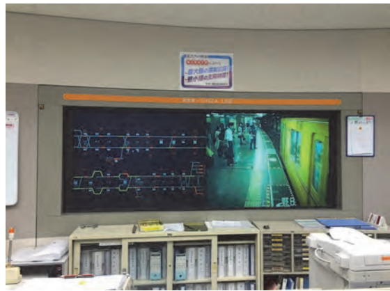
Operation Control Center 1
