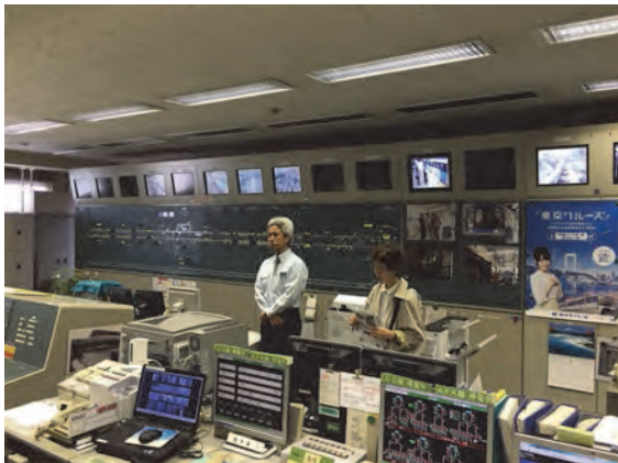
Operation Control Center 1
