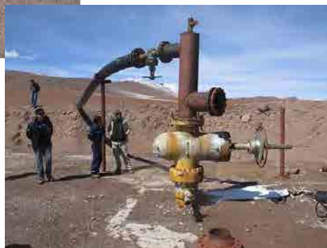
Existing well SM-4 (Reinjection well)
